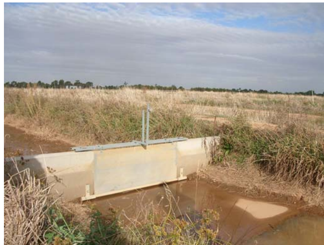
Channel stops with timers are used to regulate the height of the water
